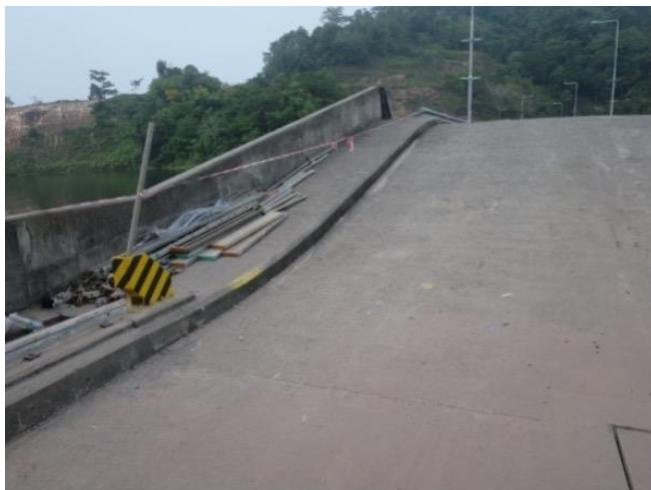
Figure 1. Detail of transition in crest elevation between concrete dam section in the foreground and rockfill dam in the background to prevent overtopping of the rockfill dam section (Kenering dam in Malaysia, a composite concrete gravity dam with two rockfill dams at abutments)
