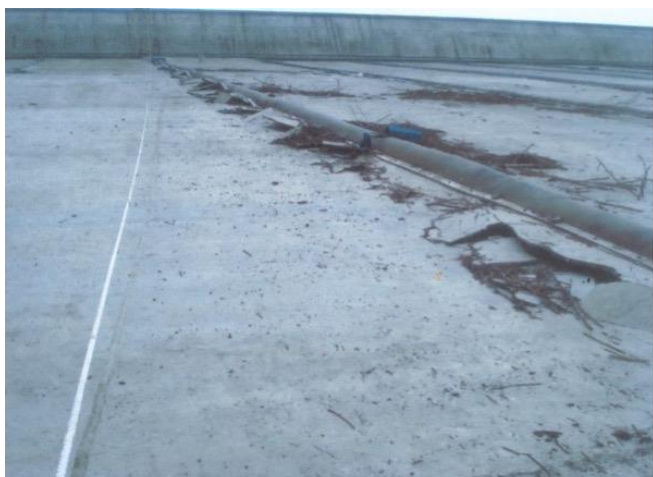
Figure 4a. Damage to vertical joint of Zipingpu CFRD caused by the 2008 Wenchuan earthquake in China (4a) and the repair of a damaged vertical joint (4b). During the earthquake the reservoir volume was about 30% of that due to normal water level (photos courtesy Xu Zeping)
