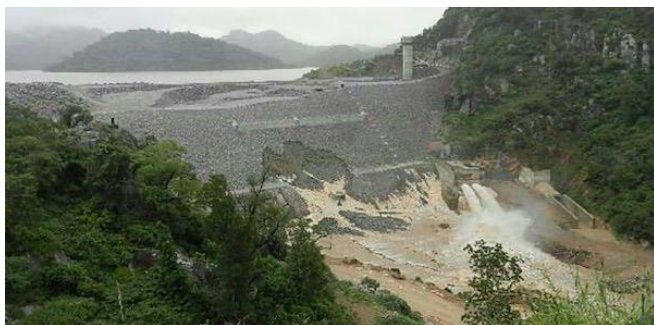
Figure 3. Seepage through Tokwe Mukosi CFRD during a severe flood in 2014 in Zimbabwe, when the dam was still under construction and the concrete face was not yet in place (CC BY 4.0)
