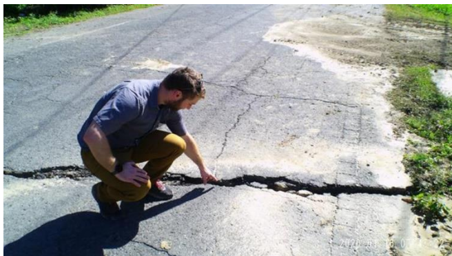
Damage from a 2020 earthquake in Puerto Rico - United States Geological Survey
