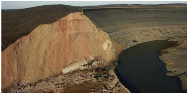
Figure 2. View of breach of shotcrete CFRD of upper reservoir of the Taum Sauk Pump Storage Plant caused by overtopping (ASDSO, 2005)
