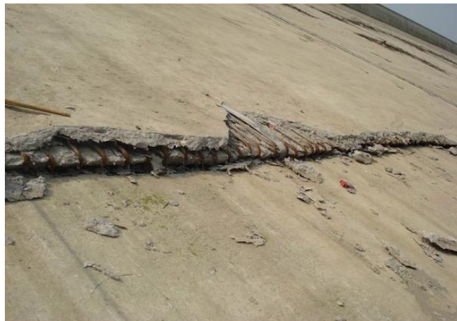
Figure 5b. Damage of horizontal joint of Zipingpu CFRD caused by the 2008 Wenchuan earthquake in China (photos courtesy Xu Zeping)
