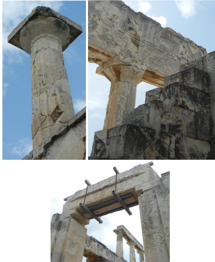
Fig. 5 Signs of visible damage in the columns of the Temple of Aphaia (top) and temporary local support measures for a cracked lintel (bottom)
